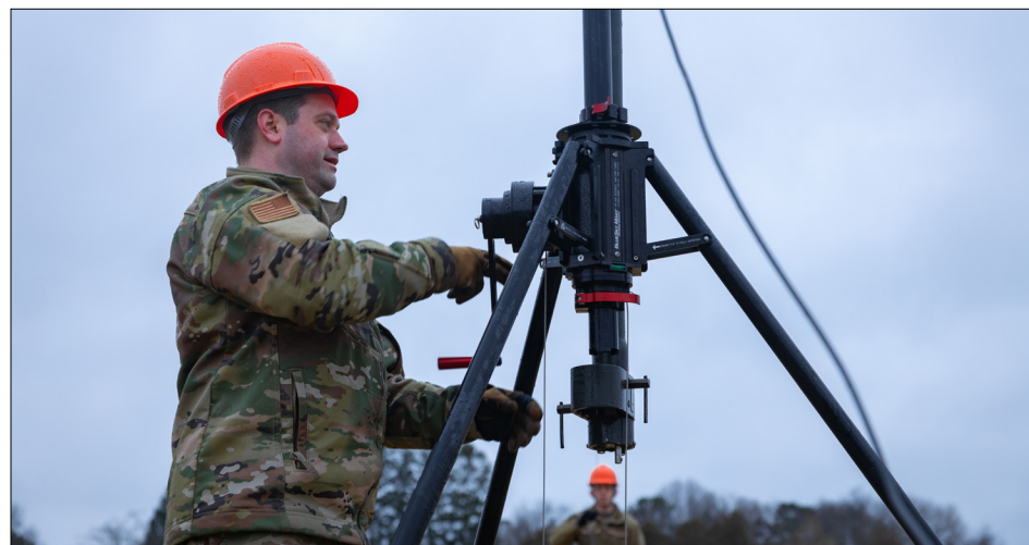
Connecticut Air National Guard Master Sgt. Jonathan Wolff, an expeditionary warfighting communications airman assigned to the 103rd Air Control Squadron, or 103rd ACS, cranks the handle of an antenna mast, part of the Tactical Operations Center - Light, or TOC-L, at Camp Nett, Niantic, Connecticut, March 5, 2024. Airmen from the 103rd ACS are conducting incremental testing of the TOC-L system for the U.S. Air Force. If adopted, this system will replace legacy command and control nodes and their respective subsystems. (U.S. Army photo by Sgt. Matthew Lucibello)
